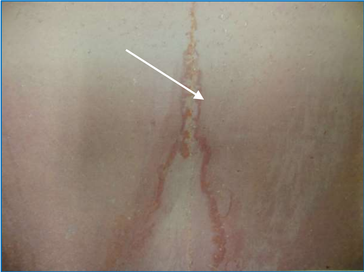
UST 89 Octane internal view: crack
