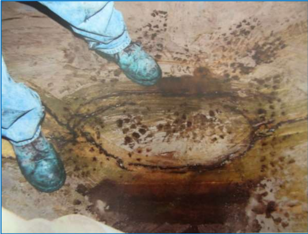
UST 92 Octane interior – cracked shell
