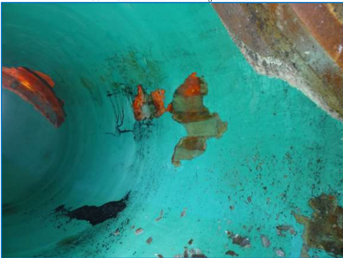
UST 92Octane interior view: lining deteriorated
