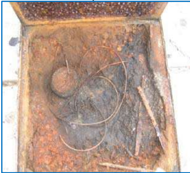
Corroded Incompatible ATG Probe
