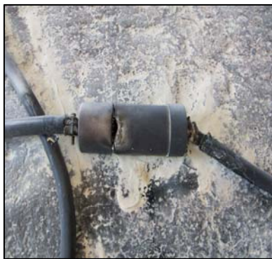
Hubbell Twist-lock 240-Volt plug & socket after incident.
