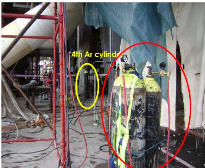
Positions of 4 Argon gas cylinders feeding inert chamber
