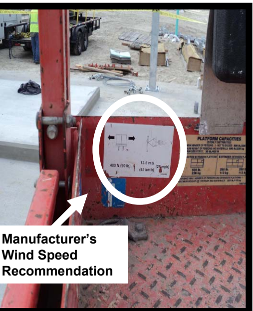
Scissor Lift in incident
